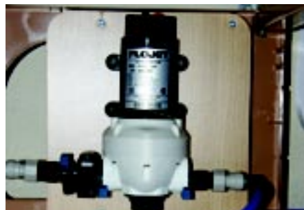
Flojet pump ensures good water distribution
