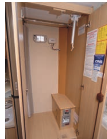
The switches are in the wardrobe, but they don't get in the way
